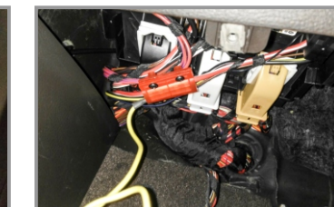
20.Our power cable is connected to the positive electrode(original power cable with red and white color), ground electrode is connected to the original ground electrode.
